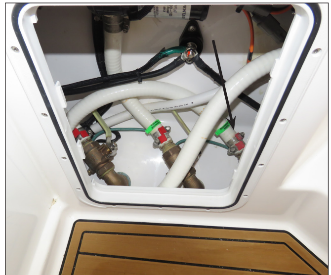
Overboard Discharge Valve
