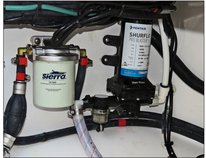
Raw Water Pressure Pump & Sea Strainer
