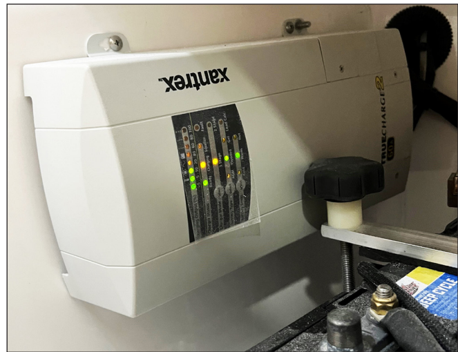
Typical Battery Charger
