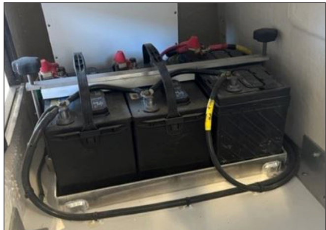
Engine & House Batteries in Compartment Below Helm Seats Boats Not Equipped with the Seakeeper
