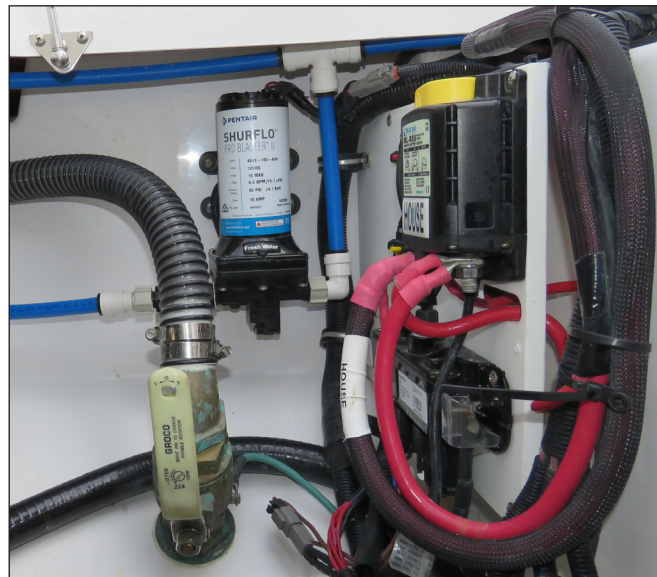
Fresh Water Pump
