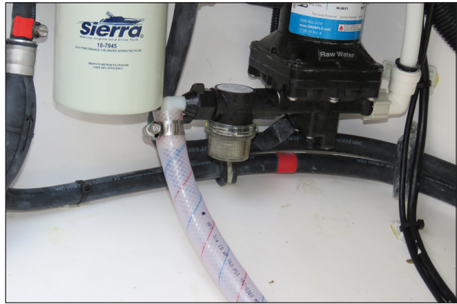
Raw Water Pump Sea Strainer
