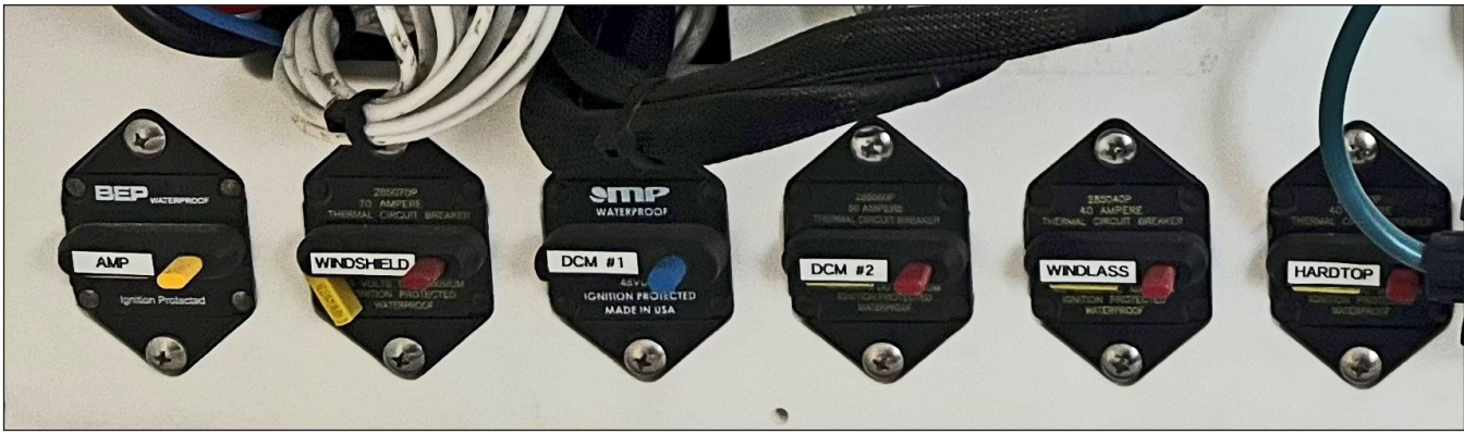
Main Circuit Breakers Behind Access Door In Aft Head Compartment
