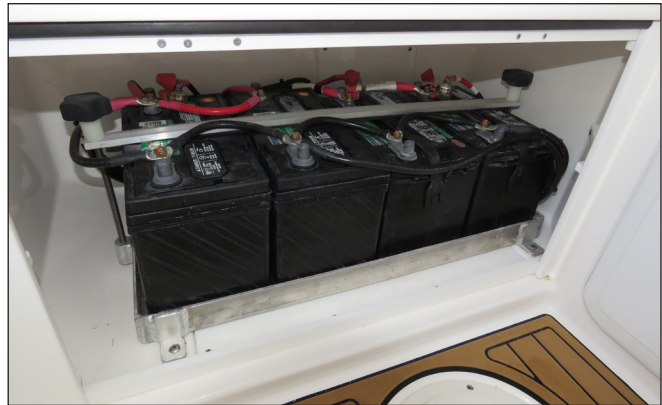
Engine & House Batteries in Forward Head Storage Compartment. Boats Equipped with the Seakeeper Option Only
