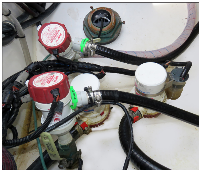
Stern Bilge Pumps & Automatic Switches
