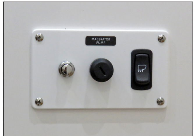
Toilet & Overboard Discharge Control Panel
