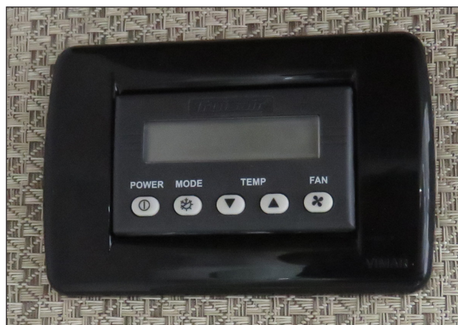
Air Conditioner Control Panel
