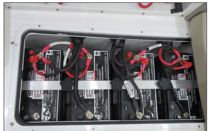
House & Optional SeaKeeper Batteries Below Port V-Berth Cushion
