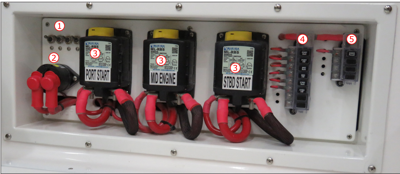
Engine Battery Switch Panel, Fuse Panels & Power Port Circuit Breakers Located Behind Port Cabin V-Berth Backrest Cushion
