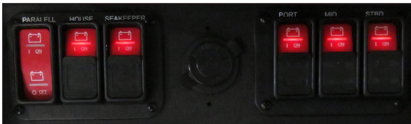
Battery Switch Panel at Helm
