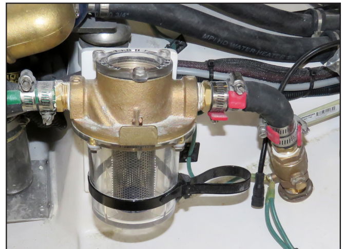
Generator Sea Strainer & Seacock
