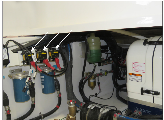
Typical Helm Master Circuit Breakers
