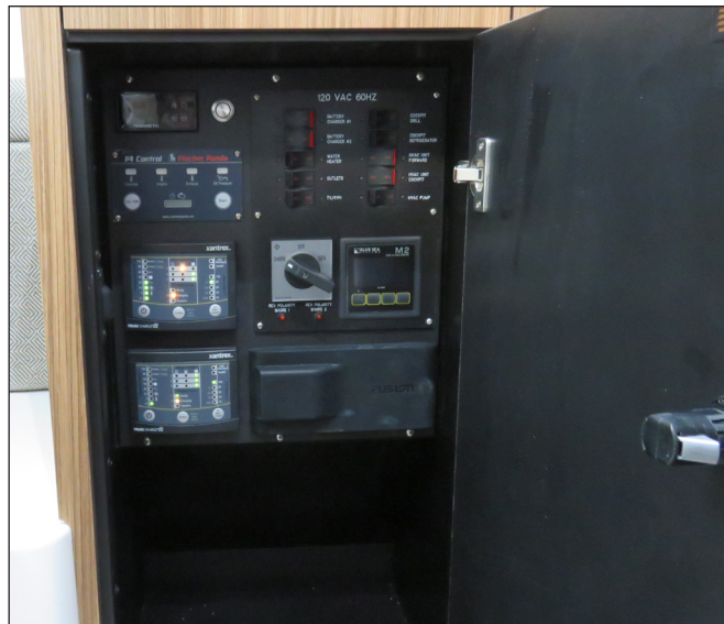
Cabin AC Electrical Panel
