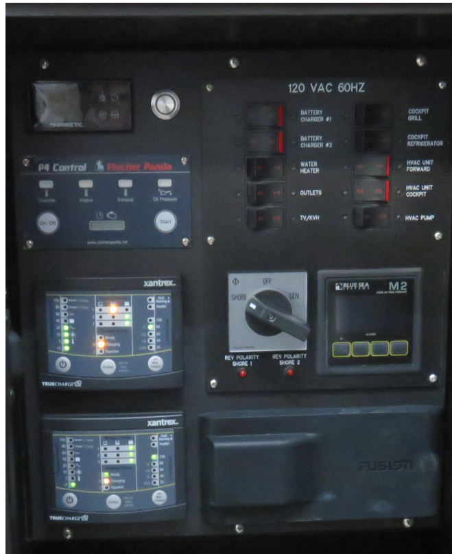
Cabin AC Panel
