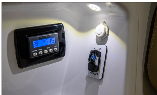
Typical Cockpit Air Conditioner Control Panel
