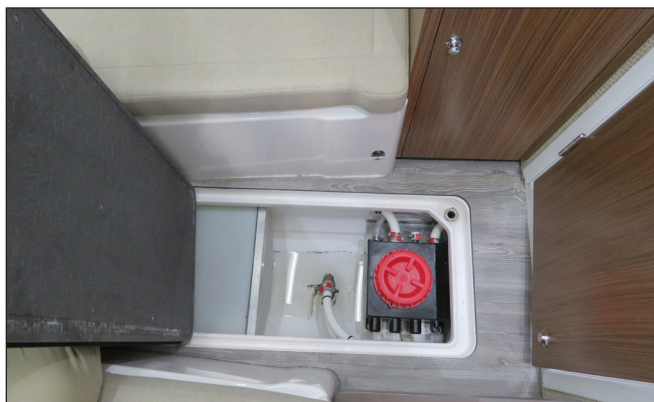
Overboard Macerator Discharge Valve
