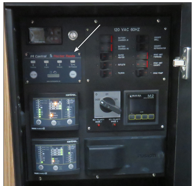
Generator Control Panel
