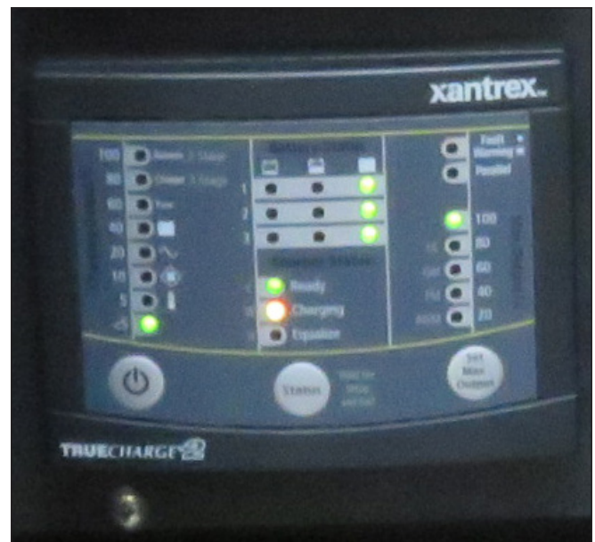
Battery Charger Control Panel & Meter in AC Panel
