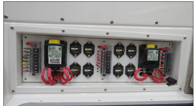
Battery Switches, Main Circuit Breakers & Continuous Power Fuse Panels
