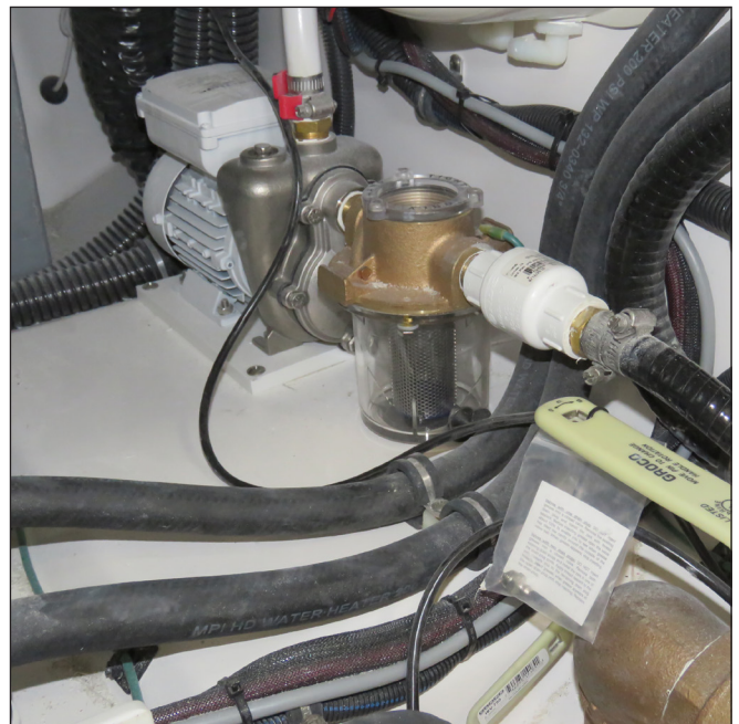
Air Conditioning Pump & Sea Strainer
