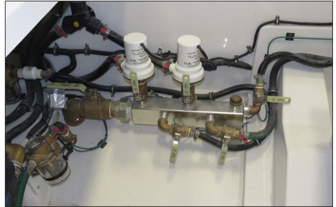
Raw Water Manifold, Port & Starboard Livewell Pumps, Raw Water Pump Connection, HVAC & SeaKeeper Pump Connections & Ball Valves
