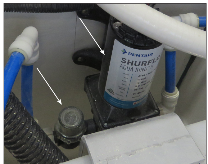
Fresh Water Pump & Strainer
