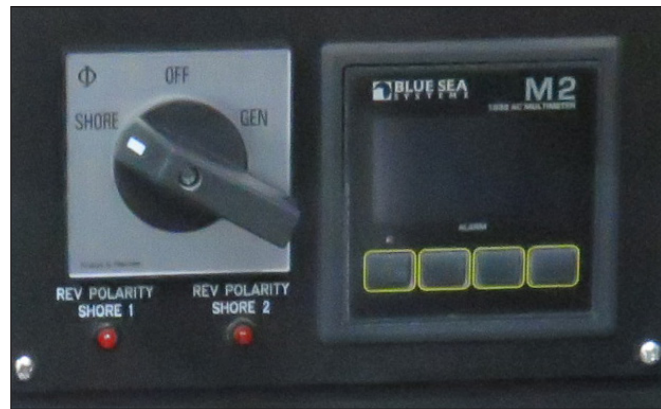
SHORE/OFF/GENERATOR Switch & Multimeter
