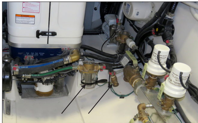
Generator Sea Strainer & Seacock Valve
