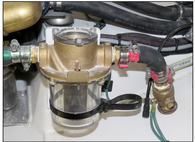
Typical Generator Seacock Valve & Sea Strainer
