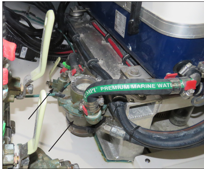
Generator Sea Strainer & Seacock Valve
