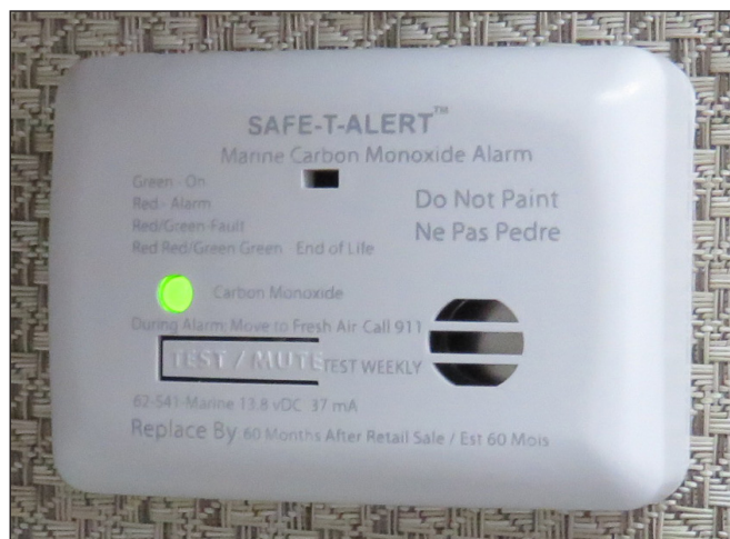
Typical Cabin Carbon Monoxide Detector
