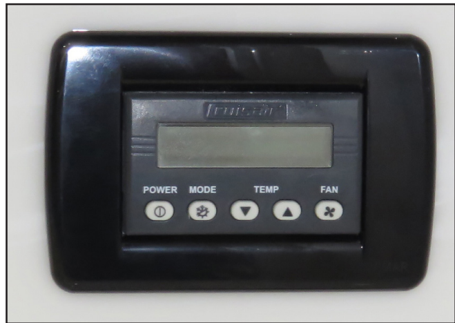
Cabin Switch Panel, HVAC Control Panel & GFI Outlet
