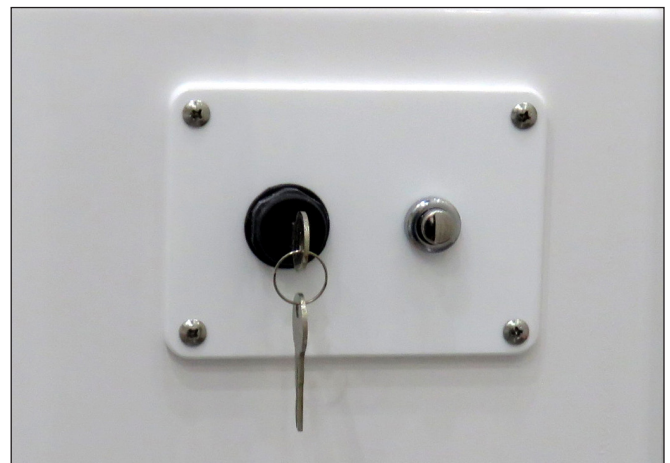
Momentary Discharge Pump Switch & Key Lockout
