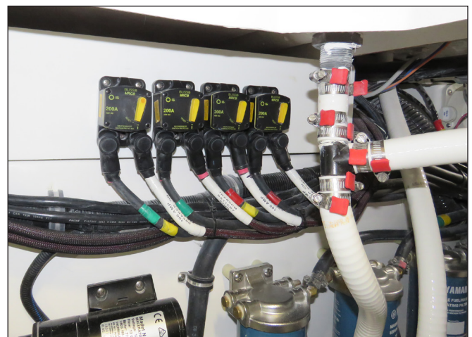
Helm Master Main Circuit Breakers
