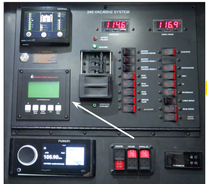
Generator Control Panel
