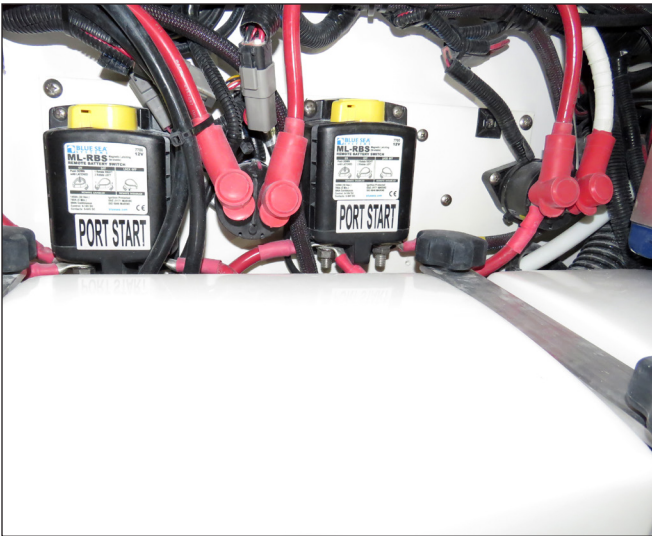
Port Engine Battery Switches & Parallel Relay in Aft Systems Compartment
