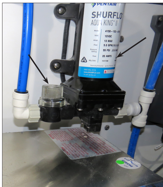
Fresh Water Pump & Strainer
