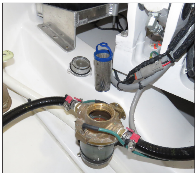
Generator, HVAC, & SeaKeeper Sea Strainer Screen & Cap
