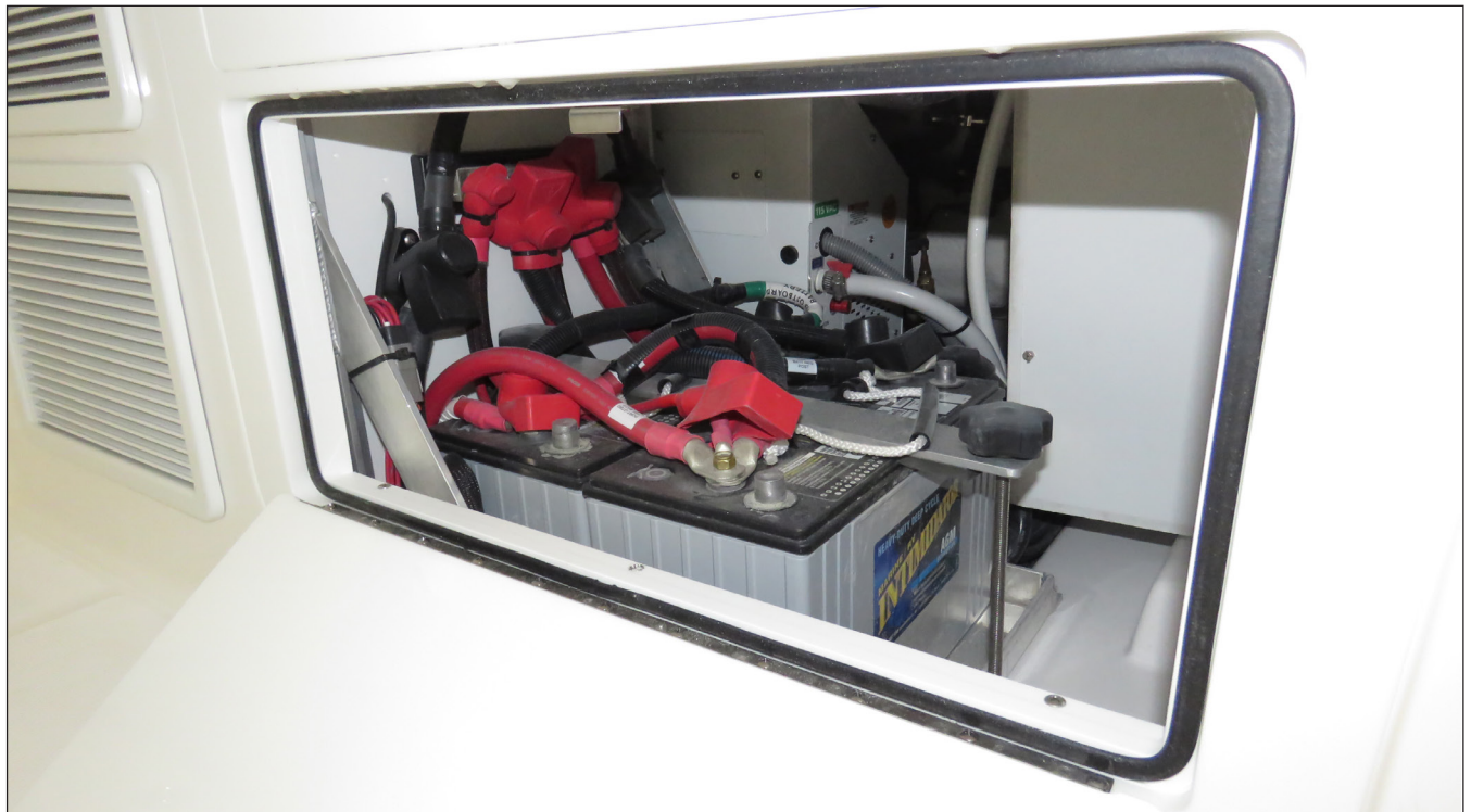
House Batteries in Mezzanine Compartment
