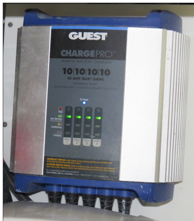
Charger for the Engine Batteries in Aft Systems Compartment
