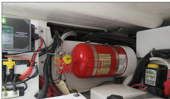
Automatic Fire Extinguishing System In The Aft Systems Compartment
