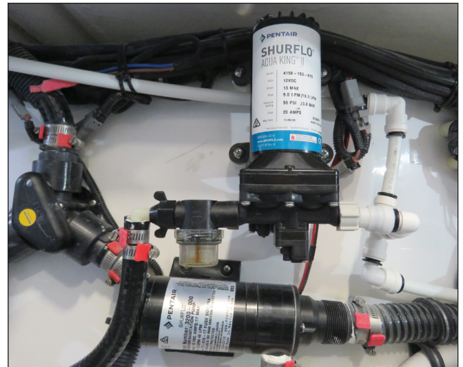
Raw Water Pressure Pump & Sea Strainer
