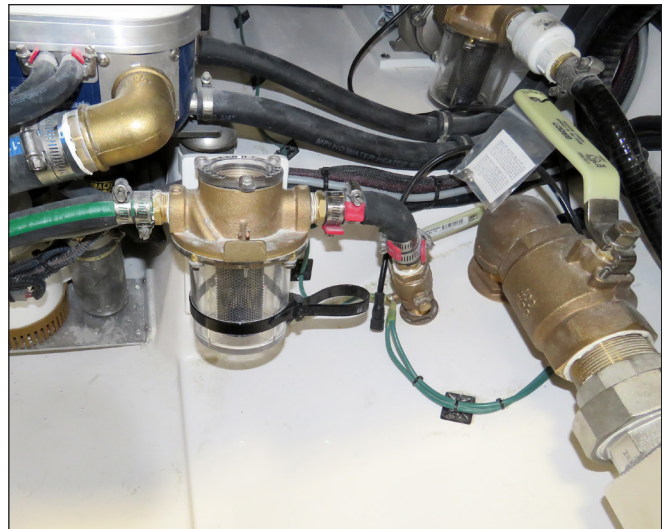
Typical Generator Raw Water Seacock & Strainer
