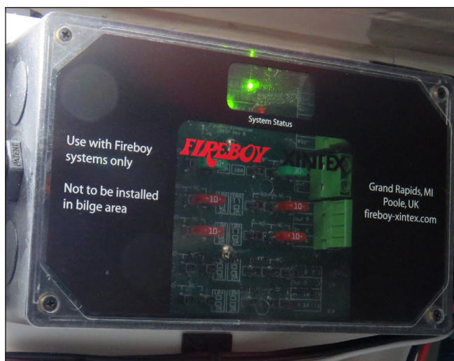
System Status Panel & Fuses
