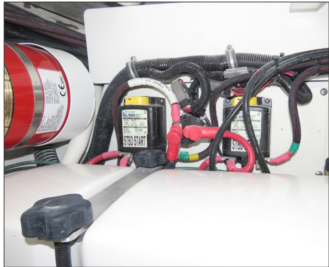
Starboard Engine Battery Switches & Parallel Relay in Aft Systems Compartment
