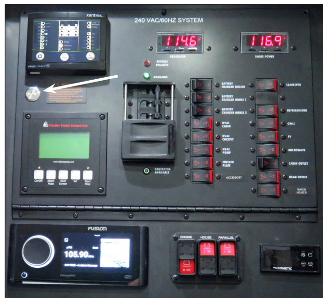
Bilge Blower Switch
