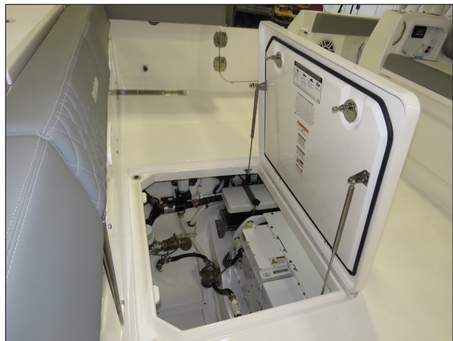
Aft Systems Compartment Hatch
