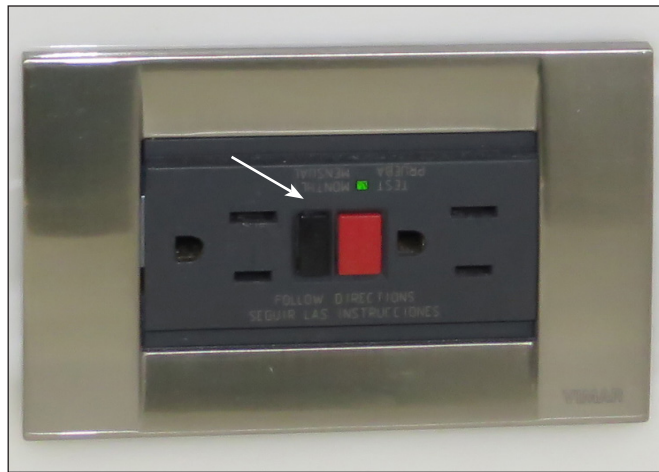
Typical GFI Outlet Test & Reset Buttons
