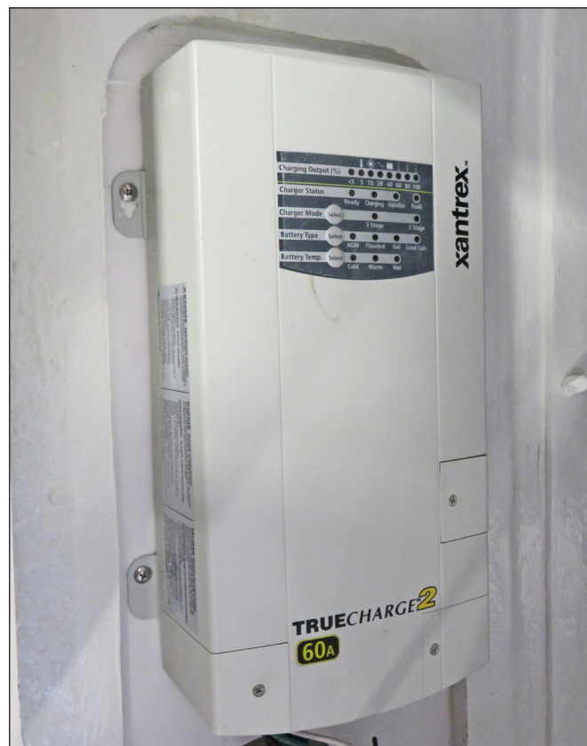
Typical House Battery Charger
