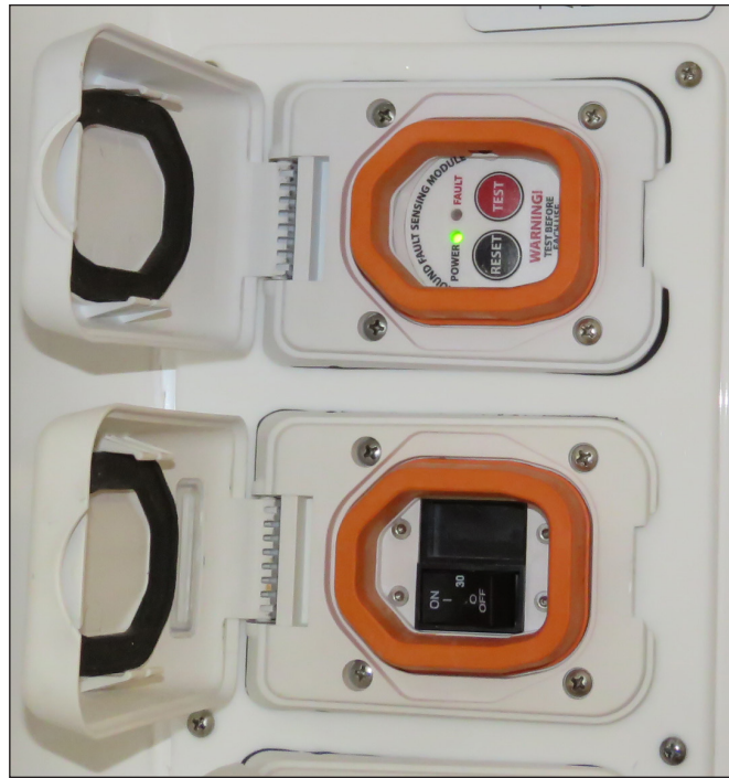
ELCI Panel & Inlet Main Breaker
