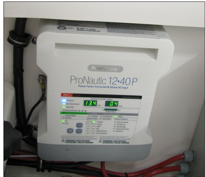
Typical Battery Charger in Systems Compartment
