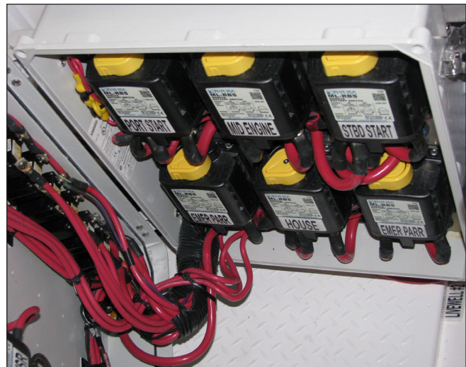
Battery Switches and Emergency Parallel Switches
