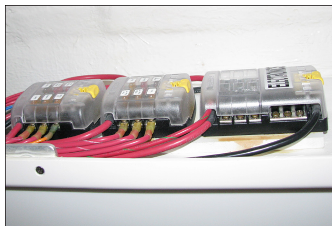
Electronics and Accessory Fuse Panels Behind Helm
