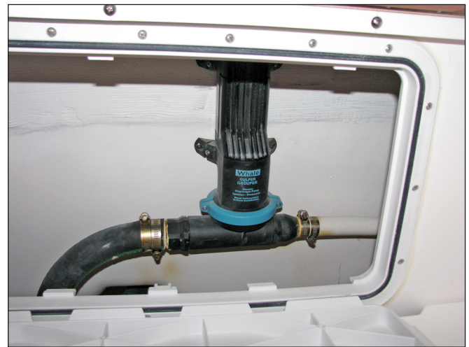
Forward Fishbox Macerator Pump Behind the Removable Hatch in the Forward Storage Compartment
