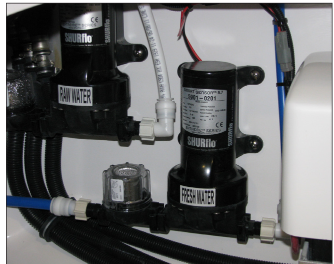
Typical Fresh Water Pump and Strainer Located in the Starboard Rear Corner of the Systems Compartment bilge
