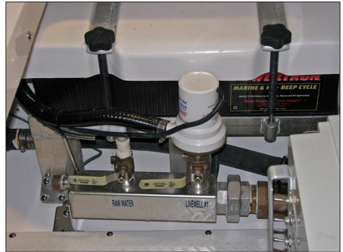
Raw Water Manifold, Livewell Pump, Raw Water Supply Pump Connection and Ball Valves
