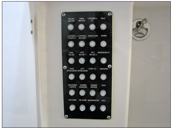
DC Circuit Breaker Panel
