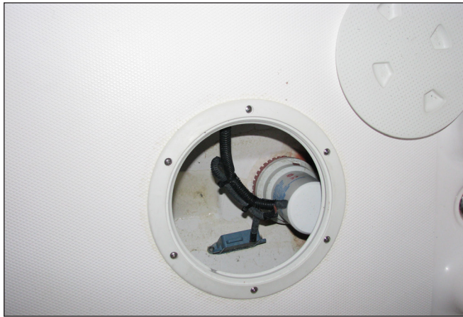
Forward Bilge Pump and Automatic Switch
