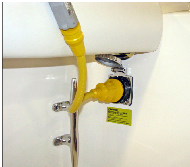
Shore Power Inlet Connection
