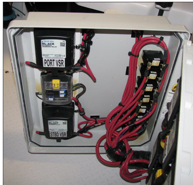
PT & STBD Voltage Sensitive Relays, Main Circuit Breakers and Continuous Power Fuse Panel
