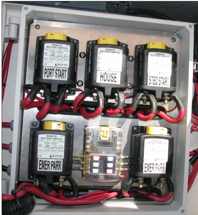
325 Center Console Battery and Emergency Parallel Switches
