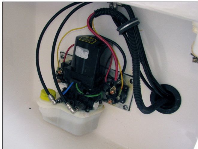
Hydraulic Pump System for Windshield In Head Compartment
