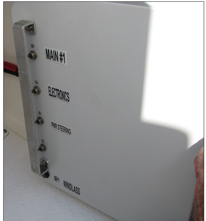
325 Center Console Main Circuit Breakers
