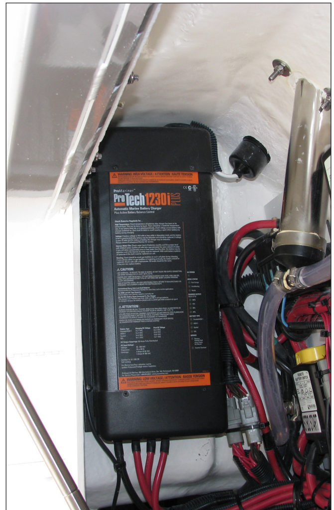
Typical Battery Charger
