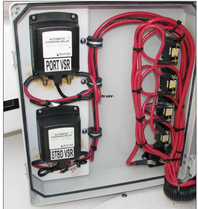
325 Center Console Voltage Sensitive Relays
