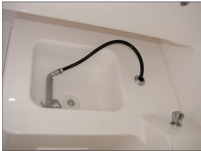
Typical Head Compartment Sink and Shower
