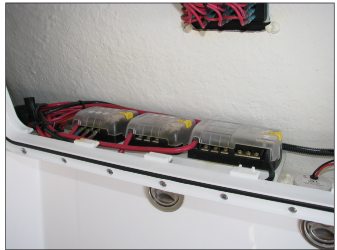
Typical Electronics and Helm Fuse Panels 325 Center Console
