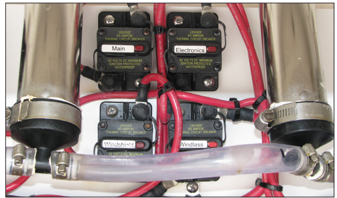
255/275/295 Center Console Main Circuit Breakers
