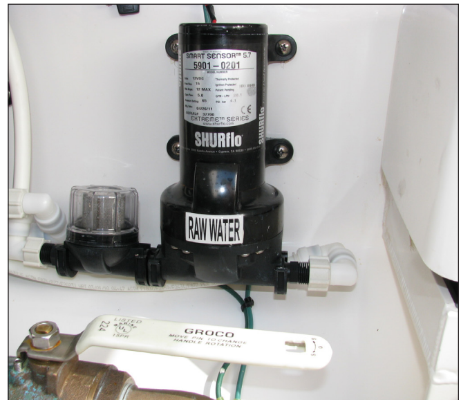
325 Center Console Raw Water Pump and Strainer
