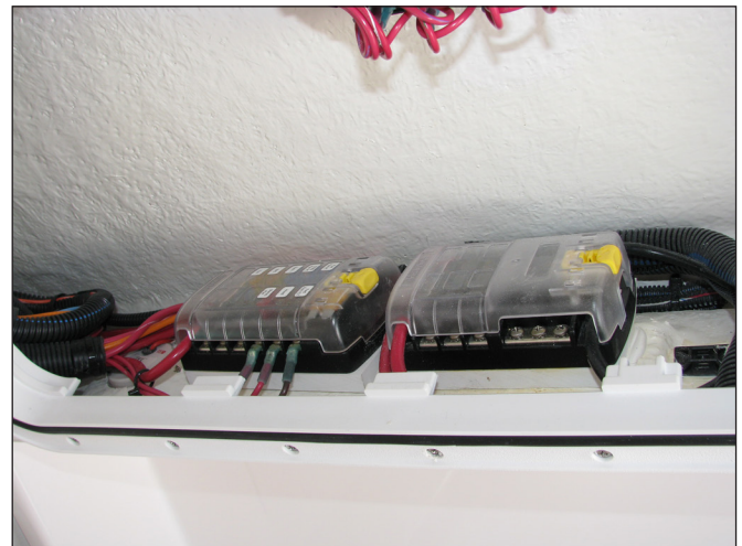
Typical Electronics and Helm Fuse Panels 255/275/295 Models
