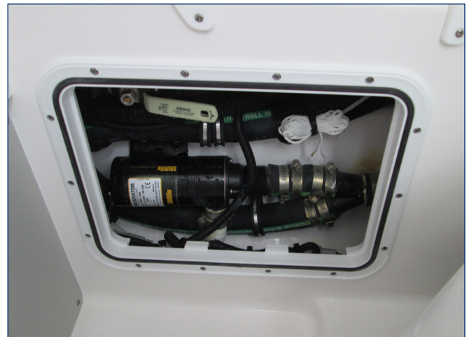
Macerator Access Hatch
