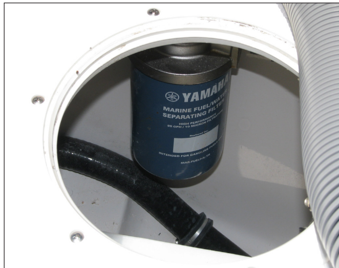
275/295 Center Console Fuel Filters Below Splashwell
