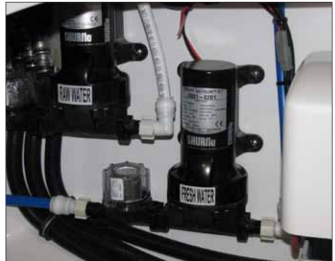
Fresh Water Pump and Strainer
