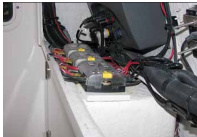
Fuse Panels Behind Helm
