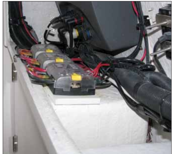
Electronics and Accessory Fuse Panels Behind Helm
