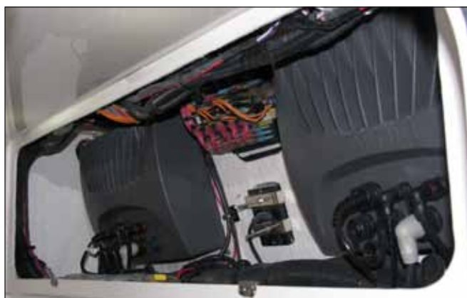
Access Behind Helm
