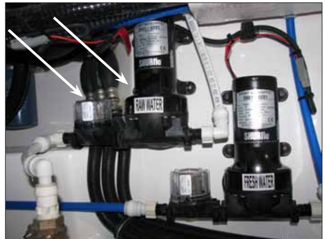
Raw Water and Fresh Water Pressure Pumps and Sea Strainers
