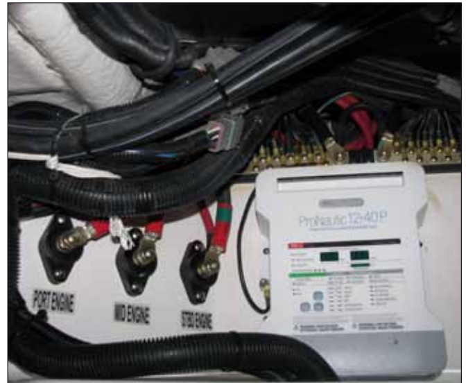
Typical Battery Charger in Systems Compartment
