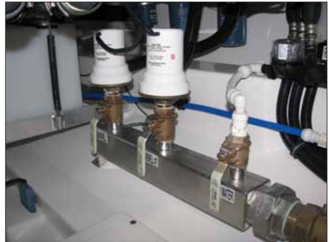
Raw Water Manifold, Livewell Pump, Baitwell Pump, Raw Water Supply Pump Connection and Ball Valves
