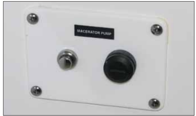
Typical Waste Discharge and Lockout Switches
