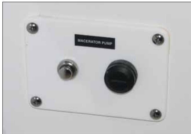
Macerator Pump Momentary Switch and Key Lockout Switch
