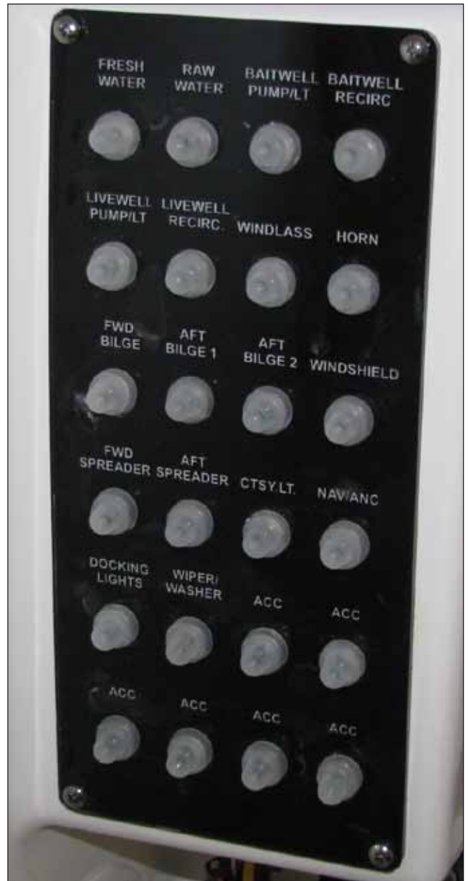
Head Compartment Circuit Breaker Panel
