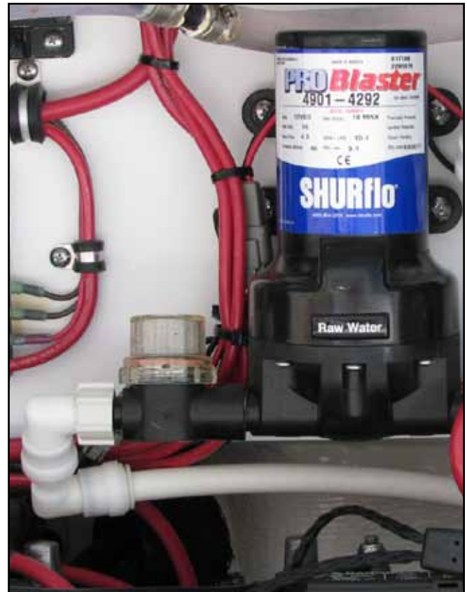
Typical Raw Water Pump and Strainer
