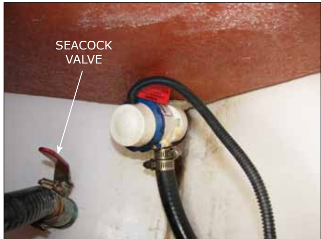
Forward Fishbox Pump Out System Hatch Drain Rail Seacock Valve
