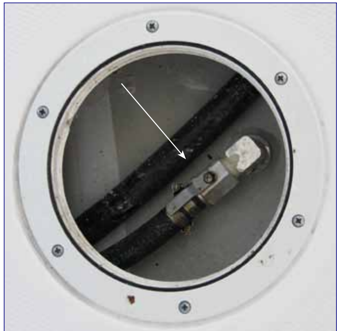
Typical Fuel Shutoff Valve
