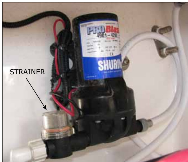
Typical Fresh Water Pump and Strainer
