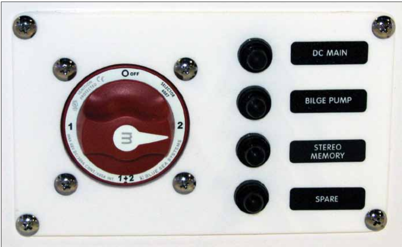
Battery Selector Switch and Circuit Breakers
