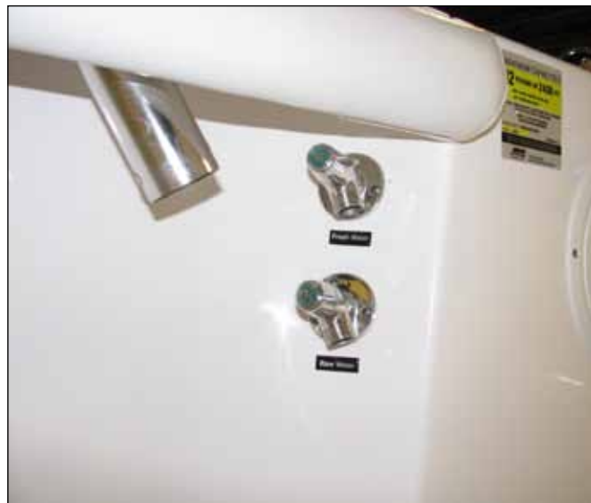
Fresh Water and Raw Water Washdown Hose Connectors
