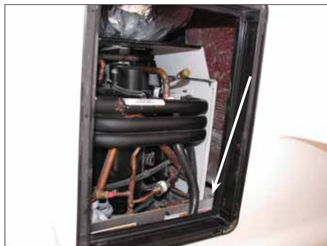
Air Conditioning Condensation Pan
