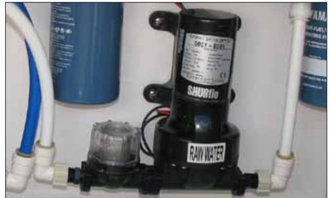
Raw Water Pressure Pump and Sea Strainer
