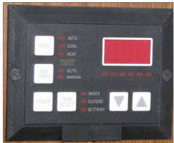
Air Conditioner Control Panel
