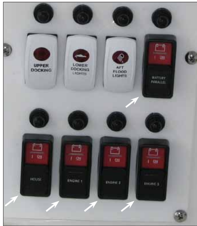
Parallel and Battery Switches
