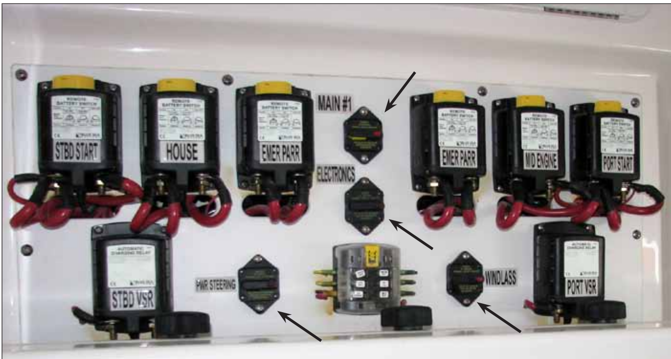
Main Circuit Breakers and Continuous Power Fuse Panel
