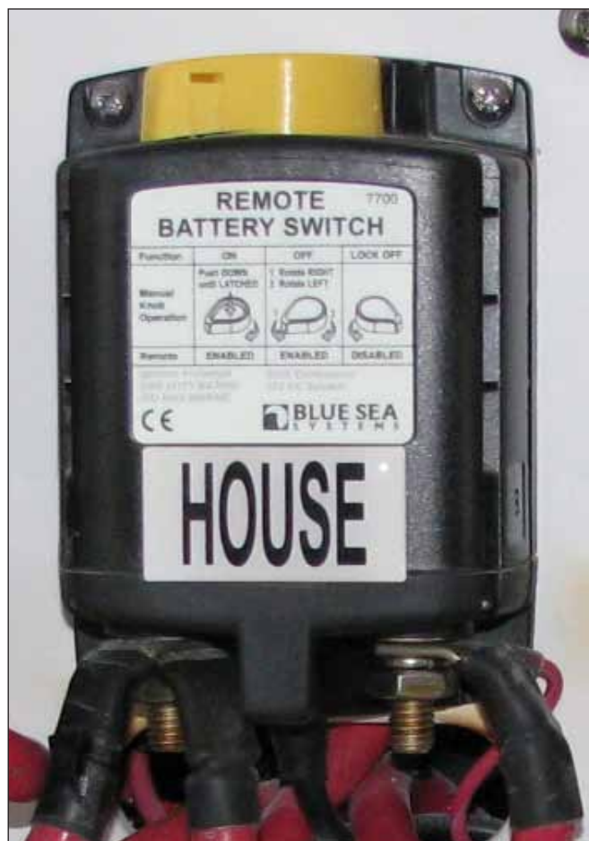
Typical Remote Battery Switch
