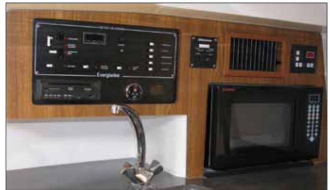
120 Volt AC Breaker Panel, Generator Control Panel and Air Conditioning Control Panel Above Gally
