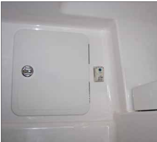
Equipment and Cabin Fuse Panel Access Door
