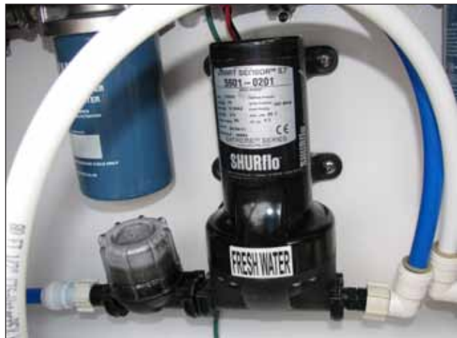
Fresh Water Pump and Strainer
