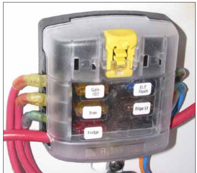
Typical Cabin DC Fuse Panel
