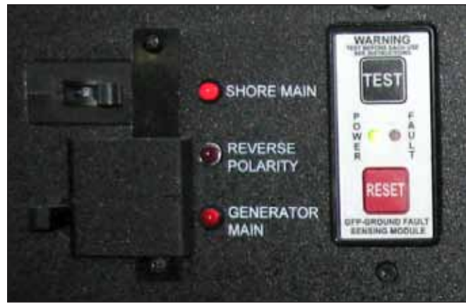
Typical Equipment Leakage Circuit Interrupter (ELCI) Shore Main Breaker, Reverse Polarity Light and Generator Main Breaker
