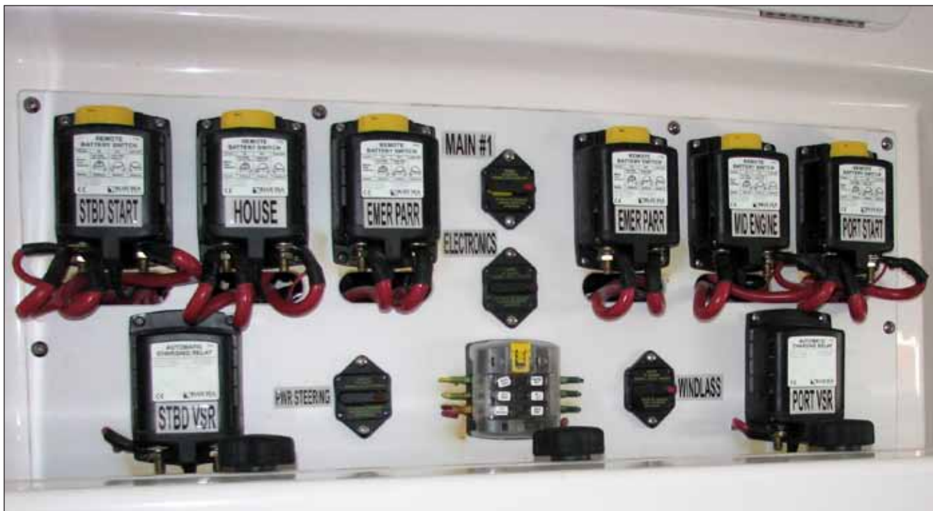
Battery Switches, Emergency Parallel Switches, PT & STBD Voltage Sensitive Relays, Main Circuit Breakers and Continuous Power Fuse Panel
