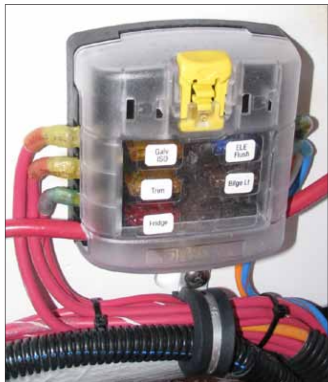
Typical DC Accessory or Electronics Fuse Panel
