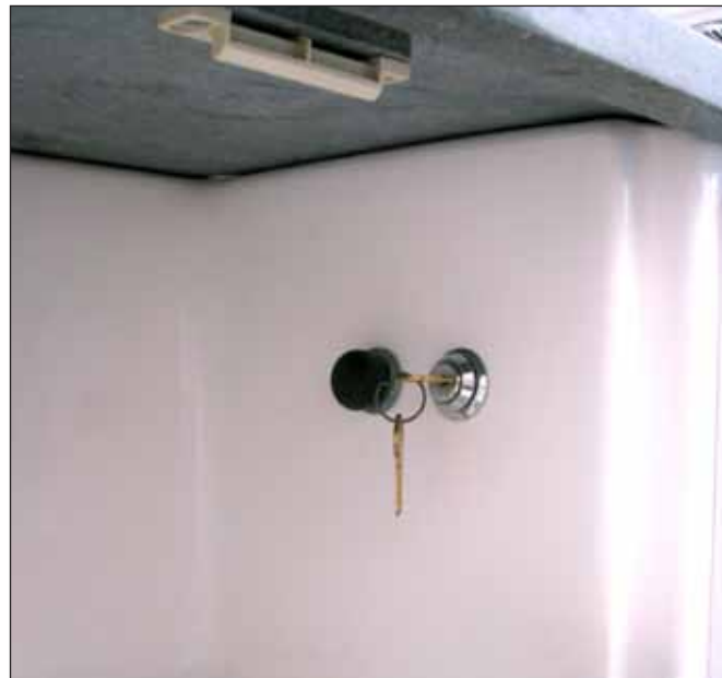
Macerator Discharge and Key Lockout Switches In Compartment Next to the Head
