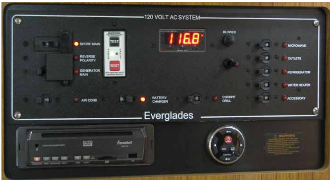
Cabin AC Circuit Breaker Panel
