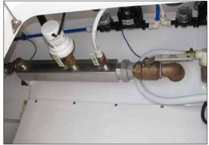
Raw Water Manifold, Livewell Pump, Raw Water Supply Pump Connections and Ball Valves
