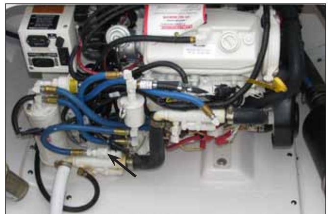
Generator In-line Fuel Filter
