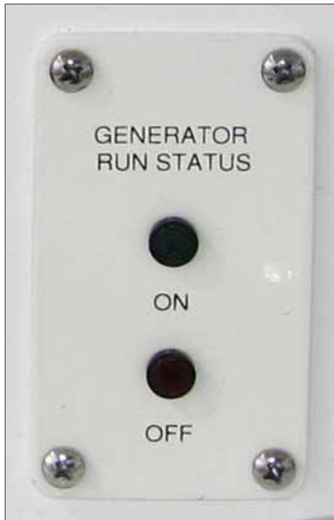
Generator Run Status Panel at the Helm
