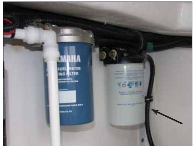
Generator Water Separator Filter
