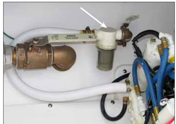
Generator Sea Strainer and Seacock Valve
