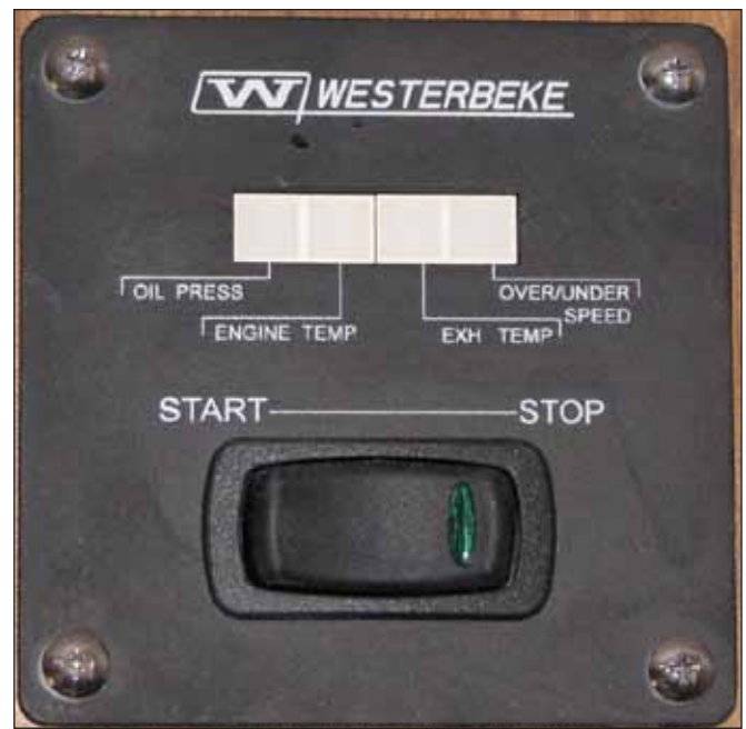
Cabin Generator Control Switch and Monitoring Lights
