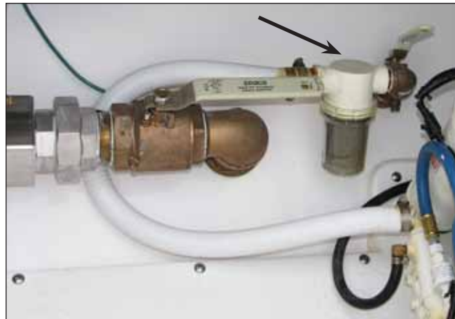
Generator Seawater Supply Seacock Valve and Water Strainer
