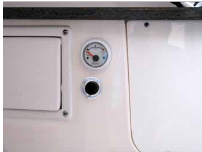
Holding Tank Gauge and Head Flush Switch
