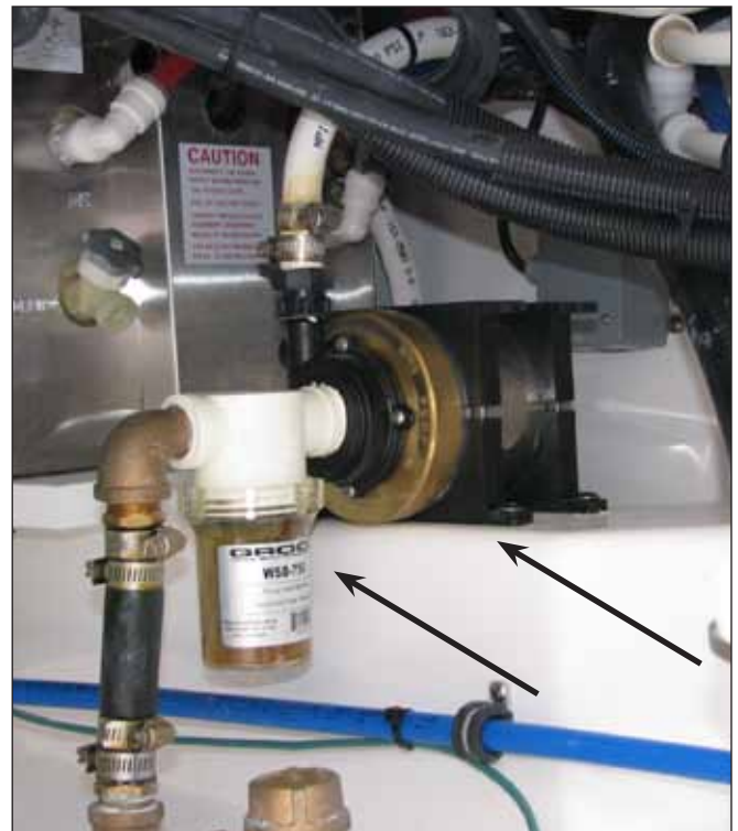
Air Conditioner Seawater Pump and Strainer
