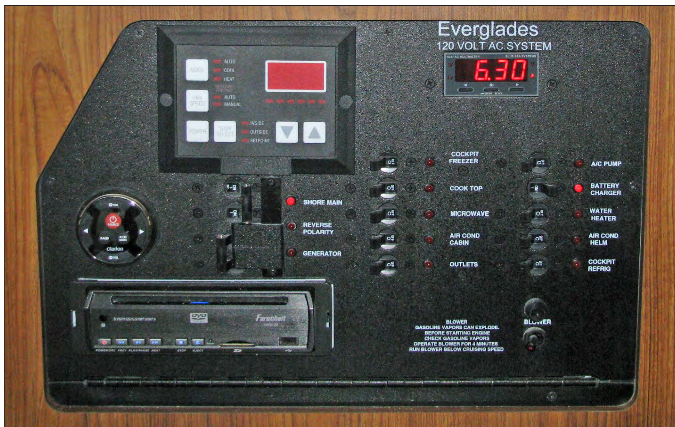
Cabin AC Circuit Breaker Panel
