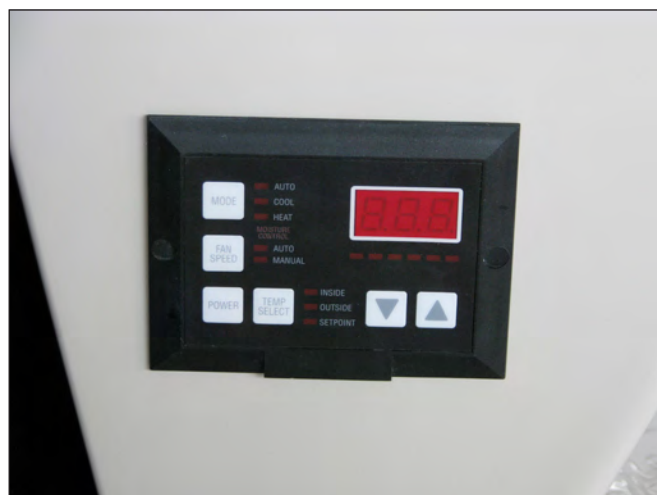
Helm Air Conditioning Control
