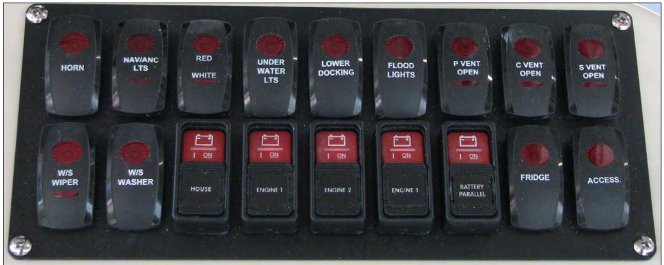
Main Accessory Switch Panel, Battery Switches and Emergency Parallel Switch in Helm
