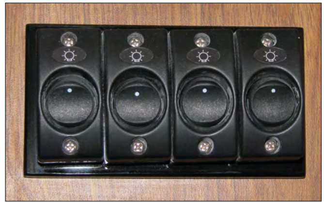
Cabin Switch Panel
