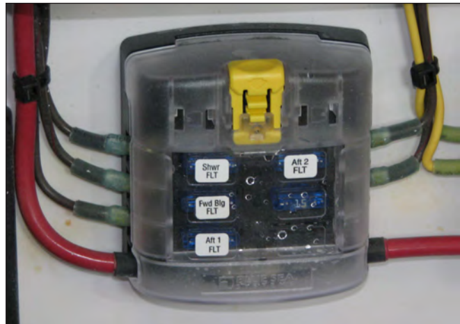
Continuous Power Fuse Panel 1
