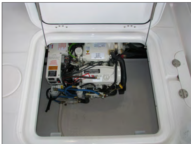
350 EX Systems Compartment Hatch
