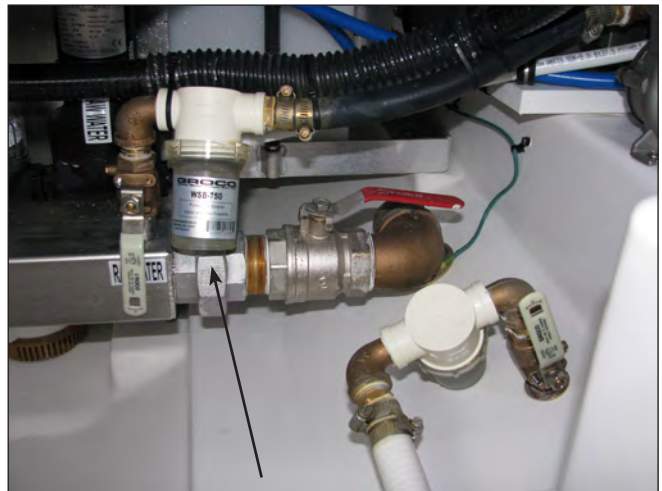
Air Conditioning Pump Sea Strainer and Valve
