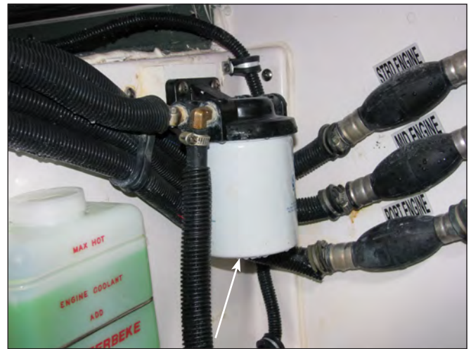
Generator Water Separator Filter
