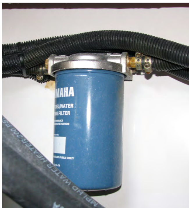
Typical Yamaha Engine Fuel Filter in Systems Compartment
