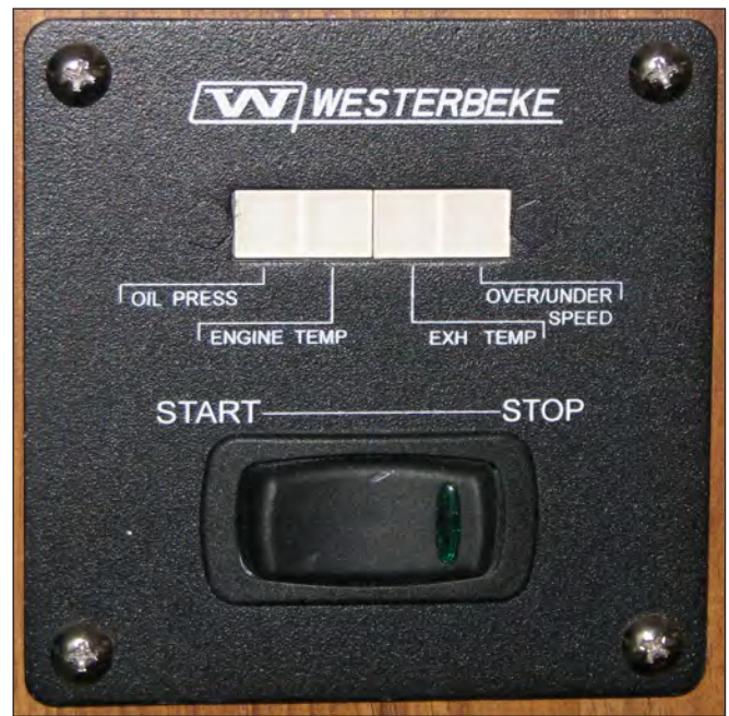
Cabin Generator Control Switch and Monitoring Lights
