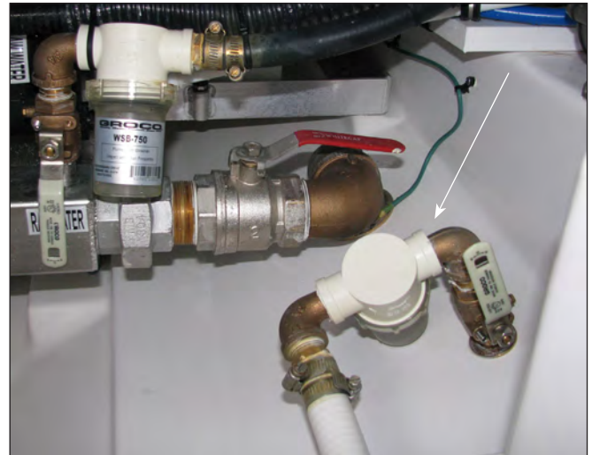
Generator Sea Strainer and Seacock Valve
