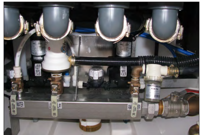
Fresh Water Pump Location in Systems Compartment
