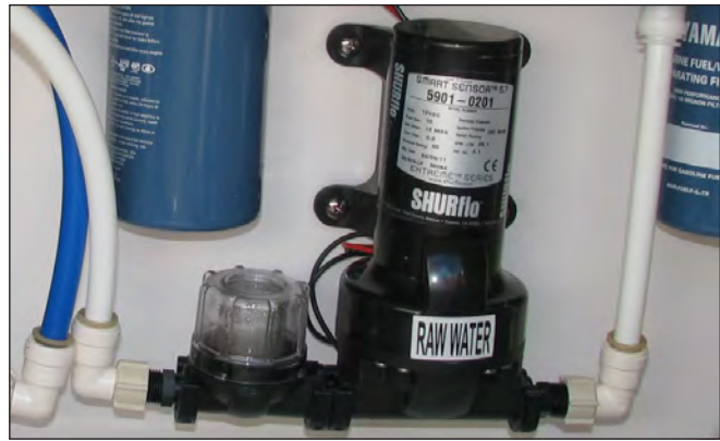
Typical Raw Water Pressure Pump and Sea Strainer
