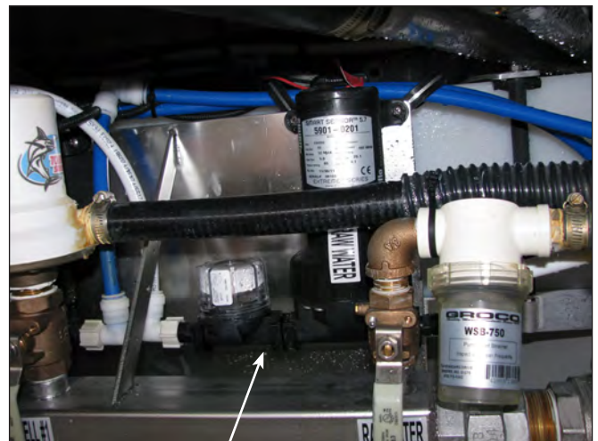
Raw Water Pump and Strainer
