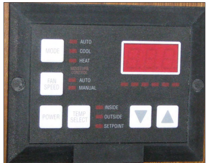
Air Conditioner Control Panel
