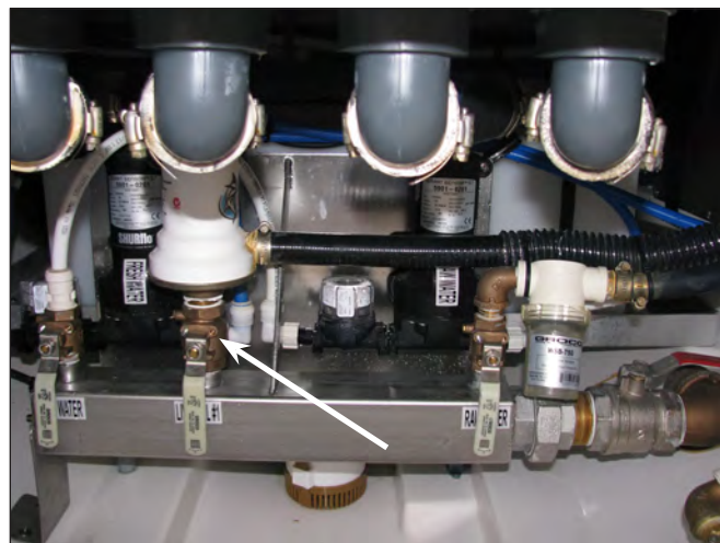
Baitwell Supply Pump and Supply Valve
