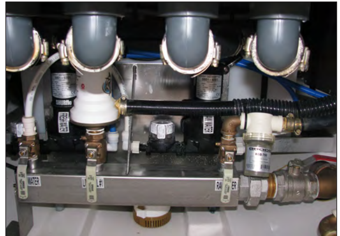
Raw Water Manifold, Baitwell Pump, Raw Water Supply Pump Connections and Ball Valves
