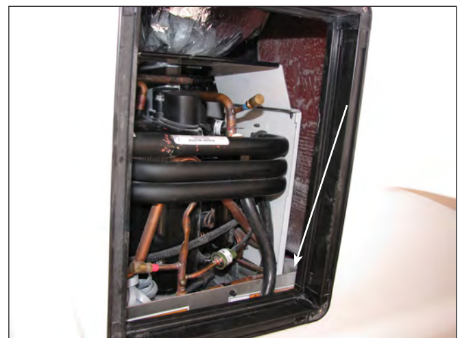
Typical Air Conditioning Condensation Pan
