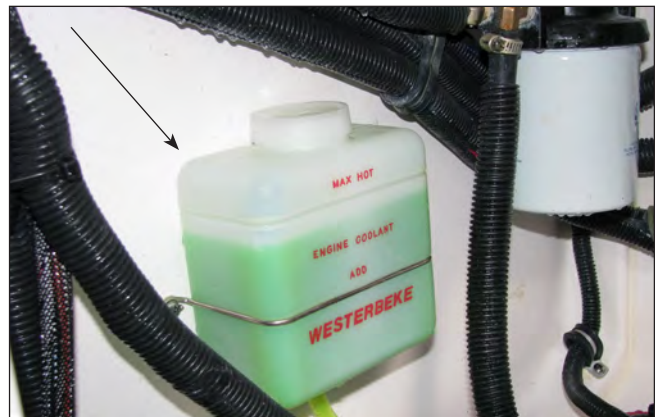
Generator Cooling System Expansion Tank
