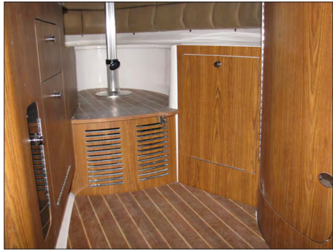
Air Conditioner in Compartment Below Table Pedestal
