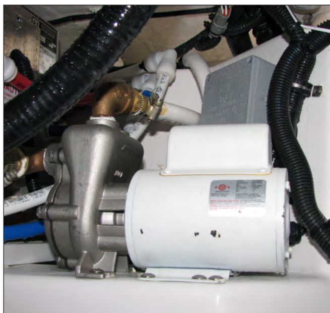
Air Conditioner Seawater Pump
