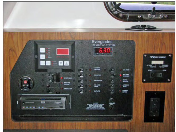
120 Volt AC Breaker Panel, Generator Control Panel and Air Conditioning Control Panel Above Gally
