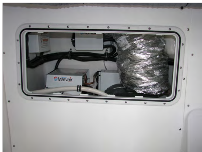
Access to Helm Air Conditioning Unit in Work Station /Tackle Storage Compartment
