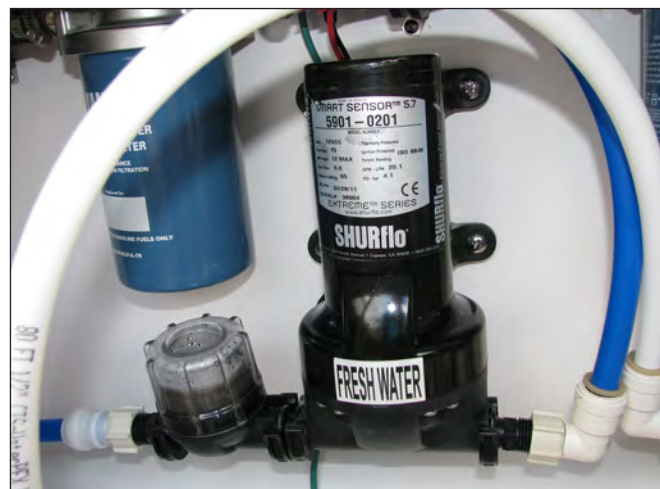
Typical Fresh Water Pump and Strainer
