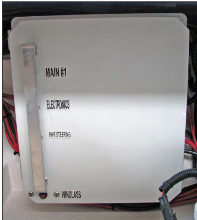
Main Circuit Breaker Panel in the Aft System Compartment
