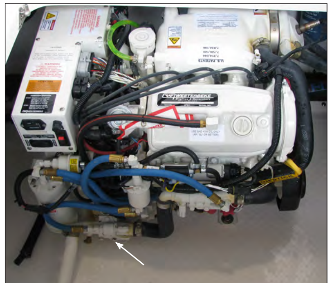
Generator In-line Fuel Filter
