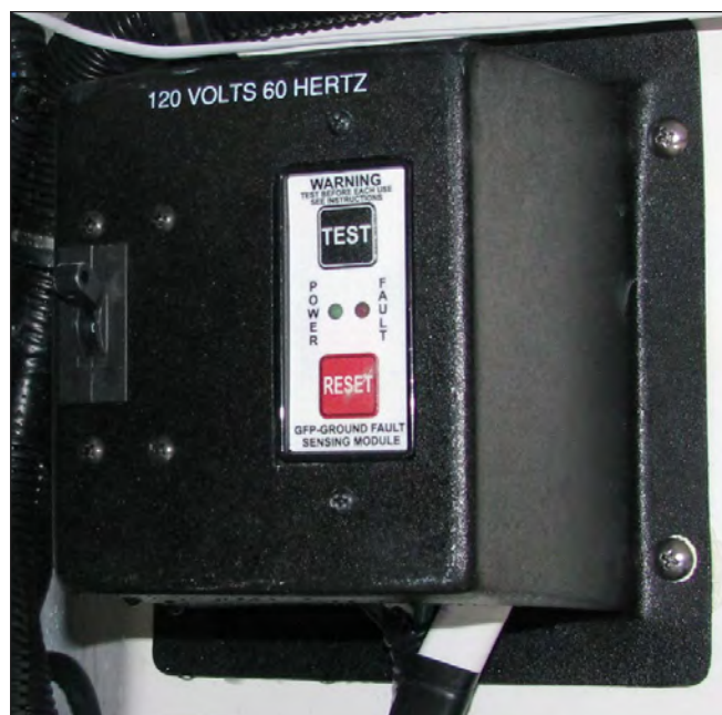
Typical Equipment Leakage Circuit Interrupter (ELCI) and Shore Main Inlet Breaker
