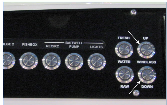
Helm Windlass Switches
