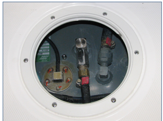
Typical Round Access Hatch In Cockpit
