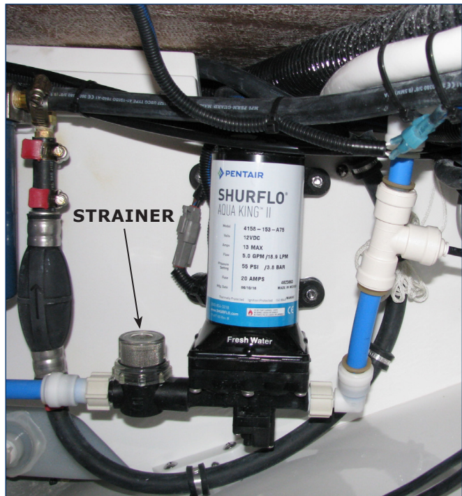
Fresh Water Pump & Strainer
