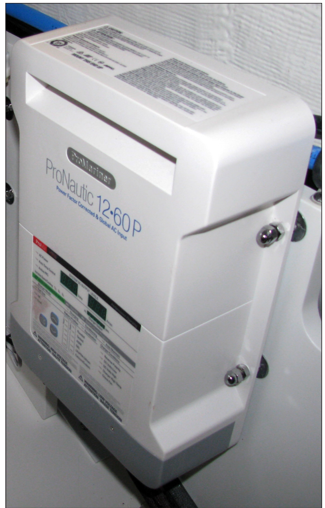
Typical Battery Charger
