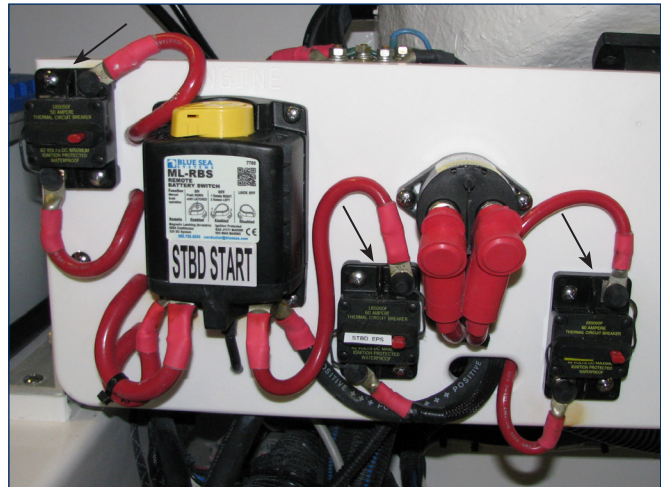
AMP & Engine Main Circuit Breakers
